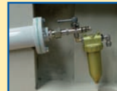
Sampled gas extraction with insulation
